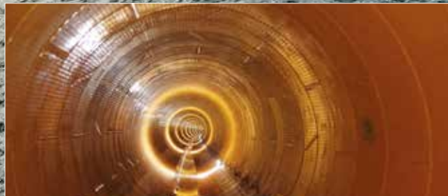
Concrete protection lining to prevent concrete deterioration of intake/discharge chambers.
