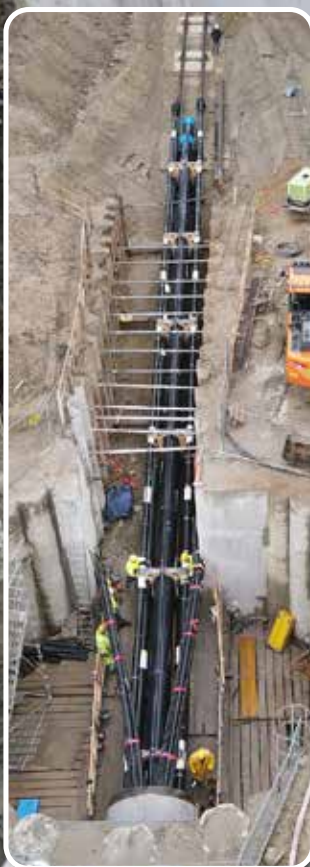
Tunneling under the Danube and laying pipelines for drinking water, natural heat, internet, electricity and gas.
